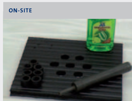
with the aid of a trepanning tool and liquid soap as lubricant
